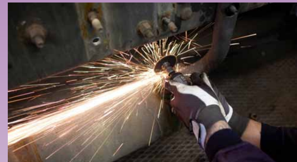
FIGURE 2 - SOME BOLTS HAVE TO BE CUT OFF. THE RUST ON THIS FH REQUIRES THE USE OF A SAW AND A WELDING TORCH.
