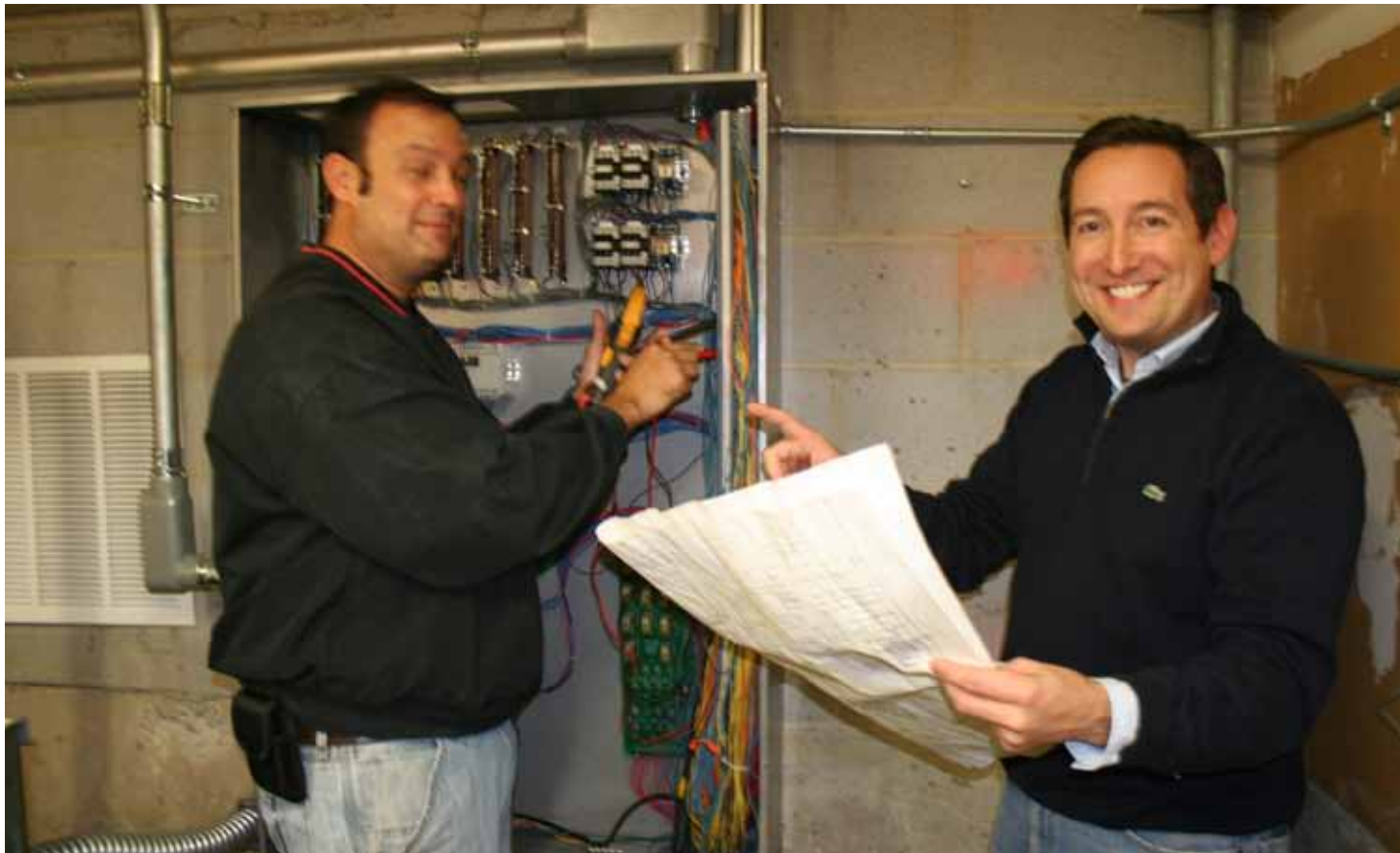
CENTURY ELEVATOR PRESIDENT JOHN POWERS (ON THE RIGHT IN BOTH) AND HIS BROTHER JEFF POWERS WORKING AT THE ELECTRICAL BOX.
