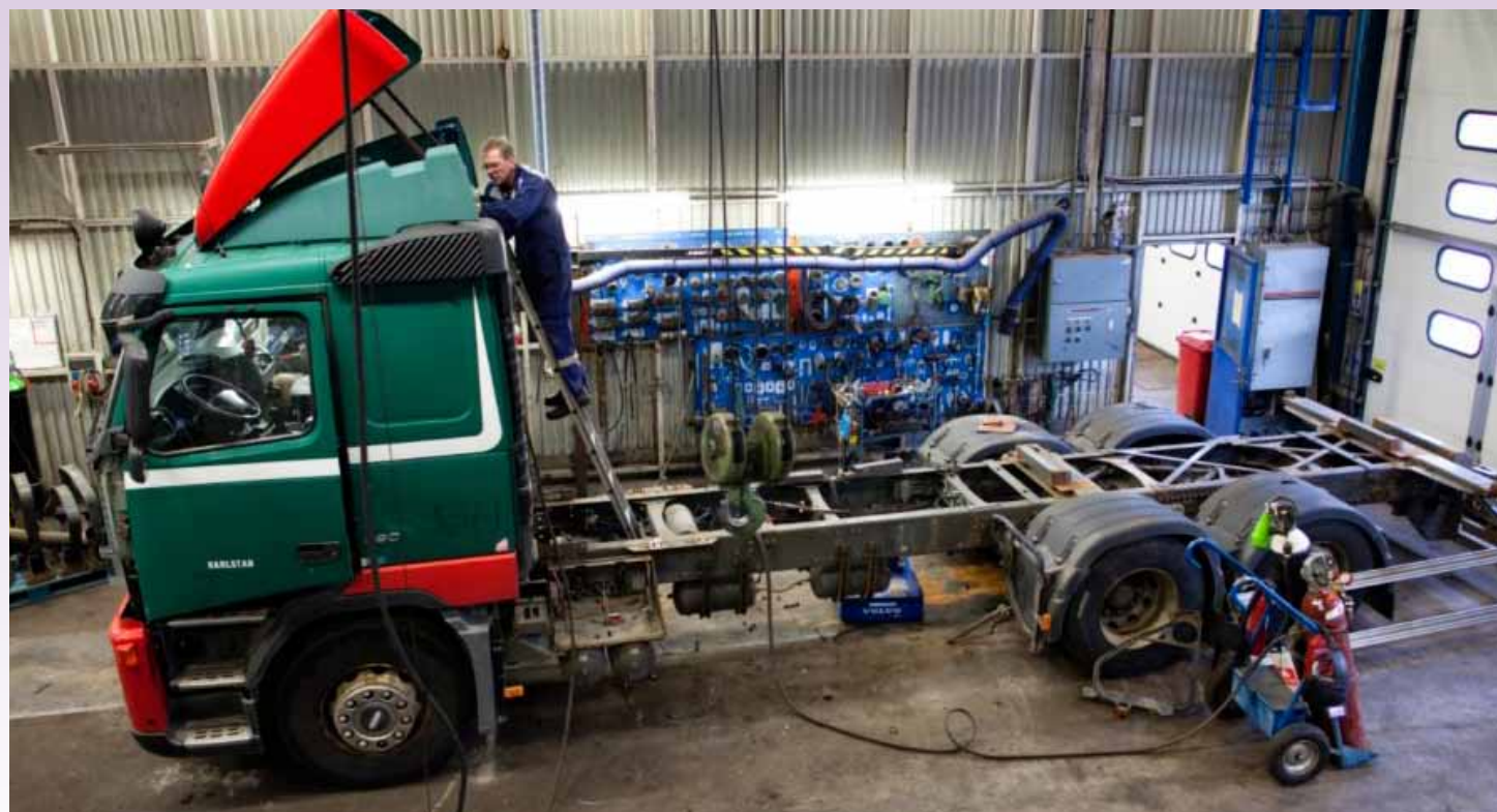
FIGURE 5 - KENNETH OLSSON REMOVES THE ROOF SPOILER. IT IS CRACKED AND WILL END UP IN THE METAL CONTAINER. THE FIRST STEP IS TO REMOVE EVERYTHING ON AND AROUND THE CAB. WITH THE SPOILER ON THE ROOF, THE CAB WOULD BE TOO TALL TO BE LIFTED OFF.
