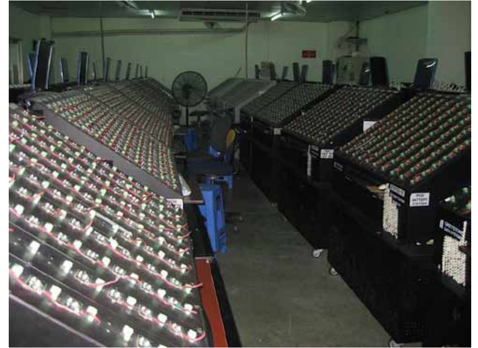
FIGURE 3: GENERIC BATTERY TESTING PROCESS
