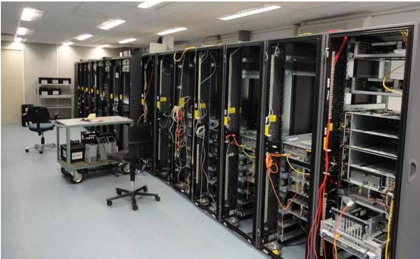
FIGURE 3: NETAPP TEST RACKS
