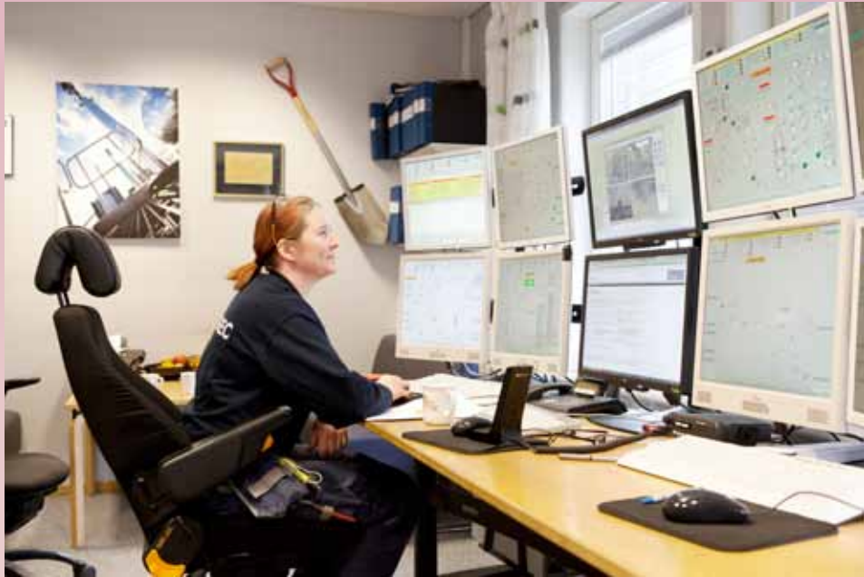
FIGURE 2: BIO-DME PRODUCTION MONITORED BY MEASUREMENT EQUIPMENT AND COMPUTER SCREENS IN THE CONTROL ROOM.
